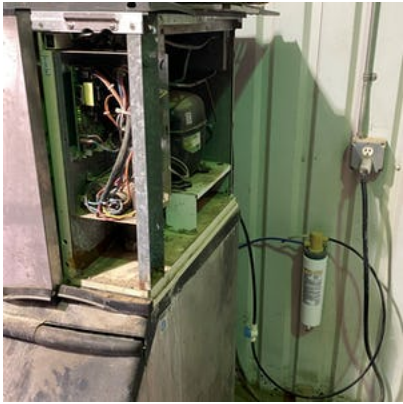
Ice machine wiring exposed post maintenance, proper lockout / tagout should be completed on any serviced machine or equipment.
