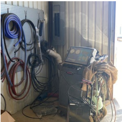
Obstructed path to breaker panel. Panel cover not closed.
