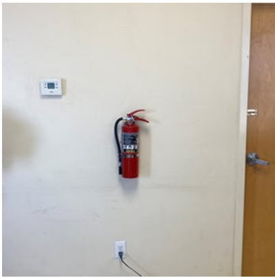
Missing location marking, will be ordered.
