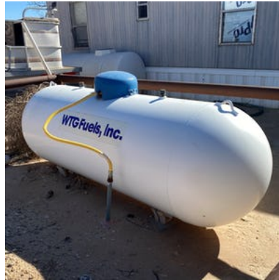
Propane storage tank for houses also missing markings and NFPA decal. Will talk to WTG about placing them on.
