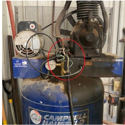
Compressor wiring exposed, needs to have the manufacturer's cover placed back on.
