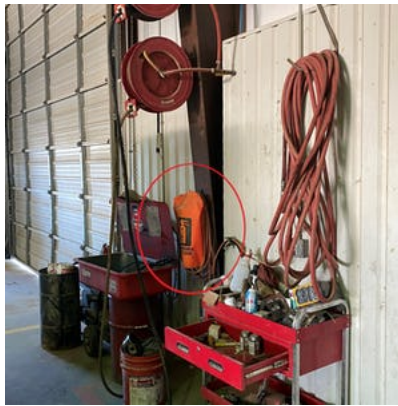
Obstructed path to extinguisher, north side of shop.
