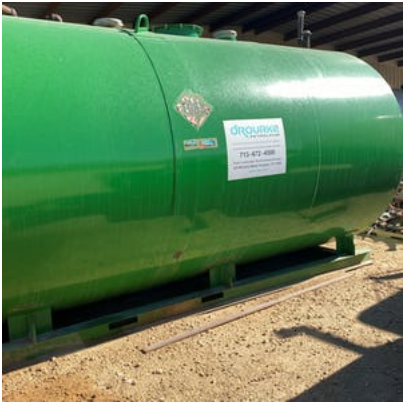
Bulk diesel tank has torn placards. Need to have O'Rourke replace them.
