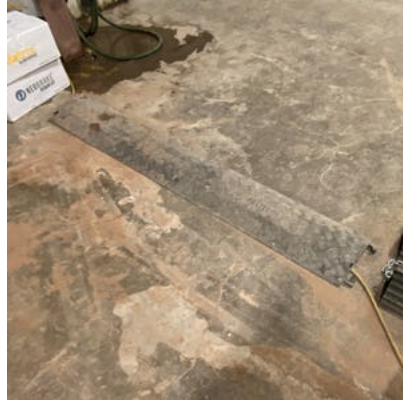
Extension cord protected in travel space.
