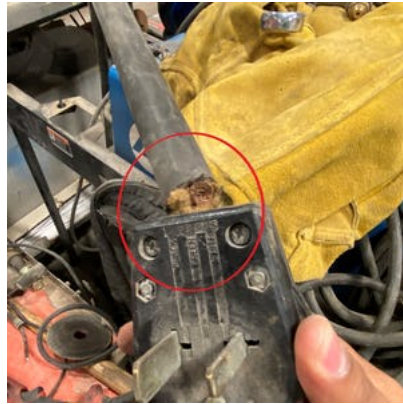
Damaged generator cord.
