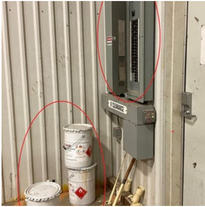
Electric breaker panel door unsecured / Incompatibility storage of flammables next to electrical sources
