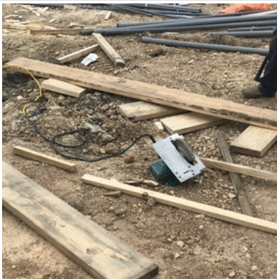
Employees were using their feet and legs to stabilize boards they were about to cut.
