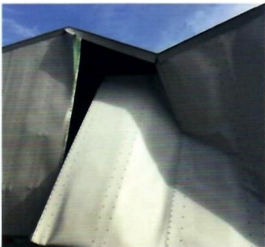
a. (1) Broken Upper Rail
