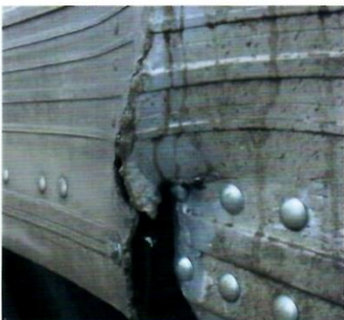
b. (1) Broken Lower Rail
