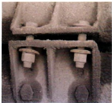
f. 25% of Anchoring Mechanisms Ineffective
