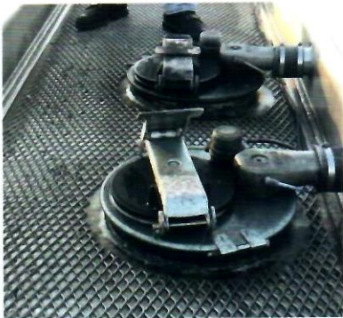
d. Manhole Cover Not Secured
