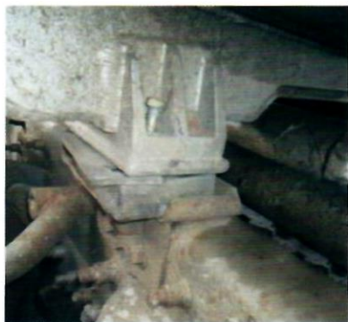
f. 25% of Anchoring Mechanisms Ineffective
