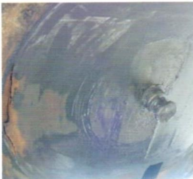
b. (5) Cracked Upper Coupler Assembly
