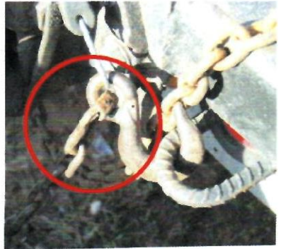
f. (4) Damaged Safety Device
