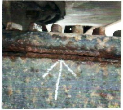
a. (2) (b) Cracked Mounting Welds
