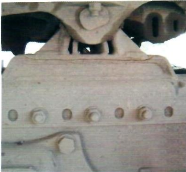
a. (2) (b) Cracked Fifth Wheel Support
