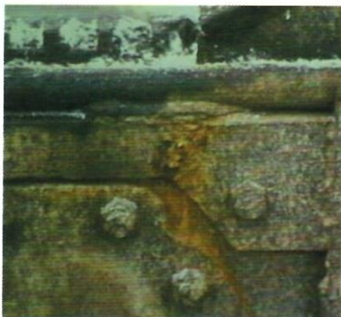
a. (2) (b) Cracked Repair Weld
