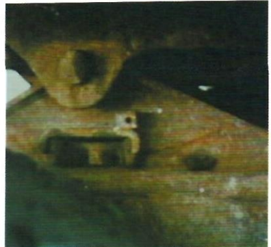
a. (2) (b) Cracked Pivot Bracket
