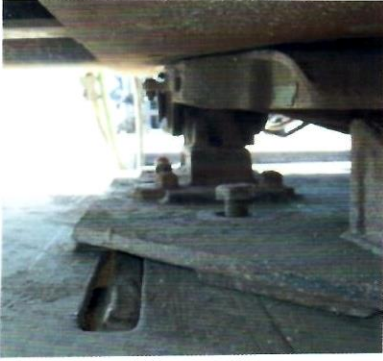
a. (2) (a) Loose Mounting Fastener
